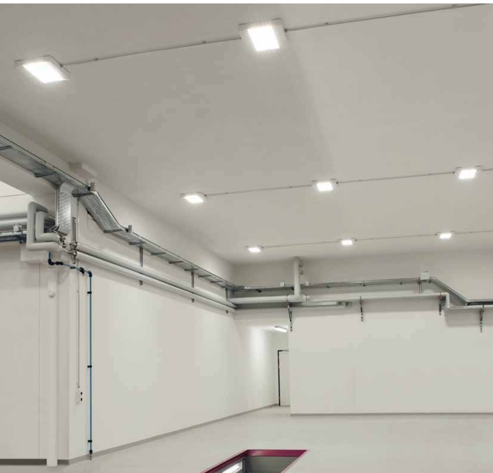
Benoil SA New building - Mendrisio - Switzerland - Architect: Studio Sangiorgio Marco SA - Electric Project: P&P Studio Elettrotecnico Sagl
